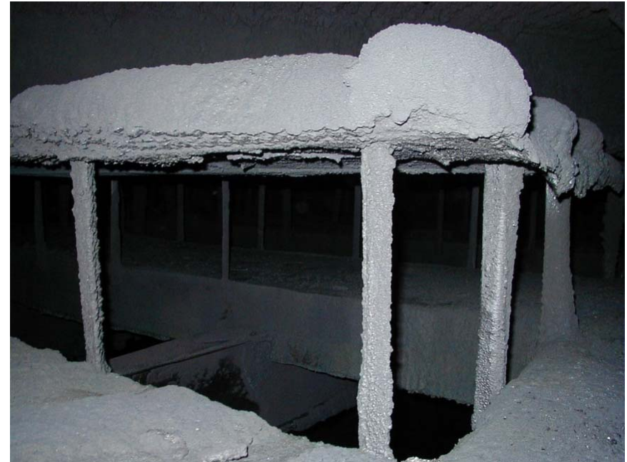
Fouled Collector Tray
